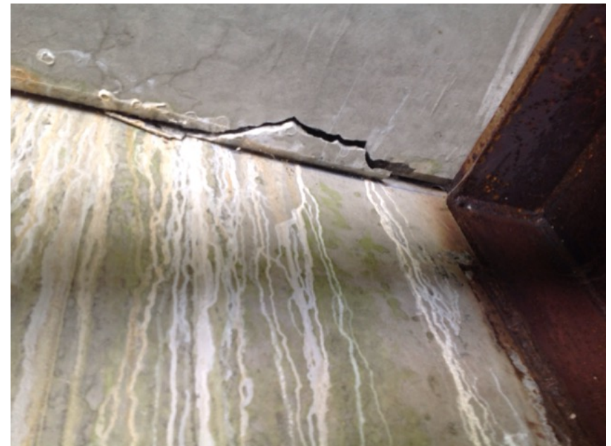
damage visible to deck from underneath
