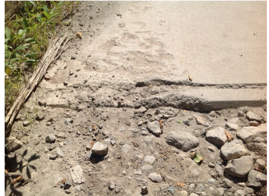
ballast wall and deck wear due to poor road conditions
